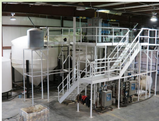
Electro Coagulation Plant Setup Operation
